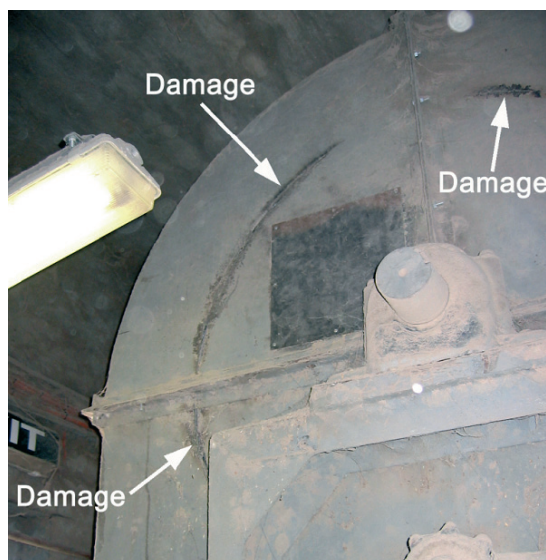
Damages that occur in a conventional bucket elevator
